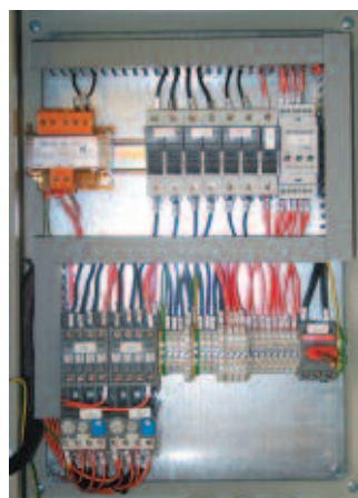
INTERNAL VIEW TWIN PUMP PANEL
