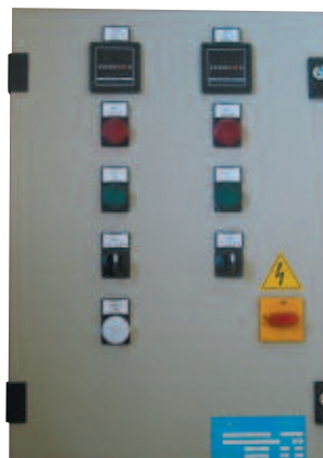
TWIN PUMP PANEL
